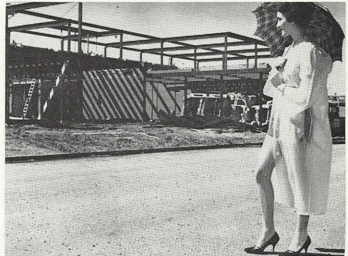
IT'S RAINING SILVER SHOWERS OF STEEL at Frontier's general office building site during the month of April. Betty Moore observes the first of the steelwork, which is now nearing completion. Although progress on the new building was temporarily waylaid because of frigid weather, workers are now taking advantage of the warm spring sun to make rapid construction advancement.
